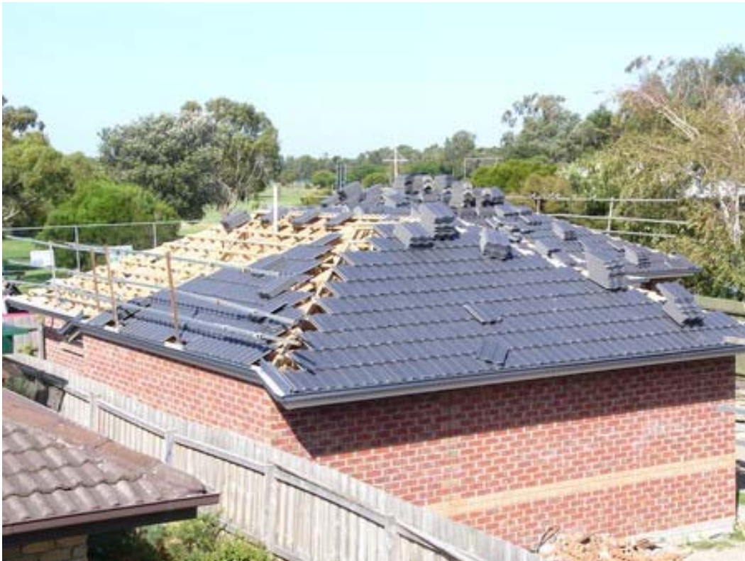
Figure 9.8.5 – Roof safety on the cheap
